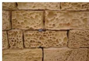
Salt weathering of stone bricks
